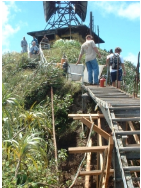
Nakoa Companies employees carry on repair Activities near the CCL building. Photo by Nakoa Companies
